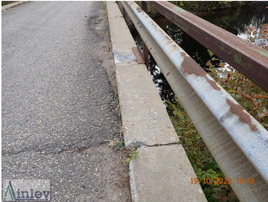
Photo 9: West Curb – Light Scaling Throughout, Localized Medium Spalls and Medium to Wide Cracks
