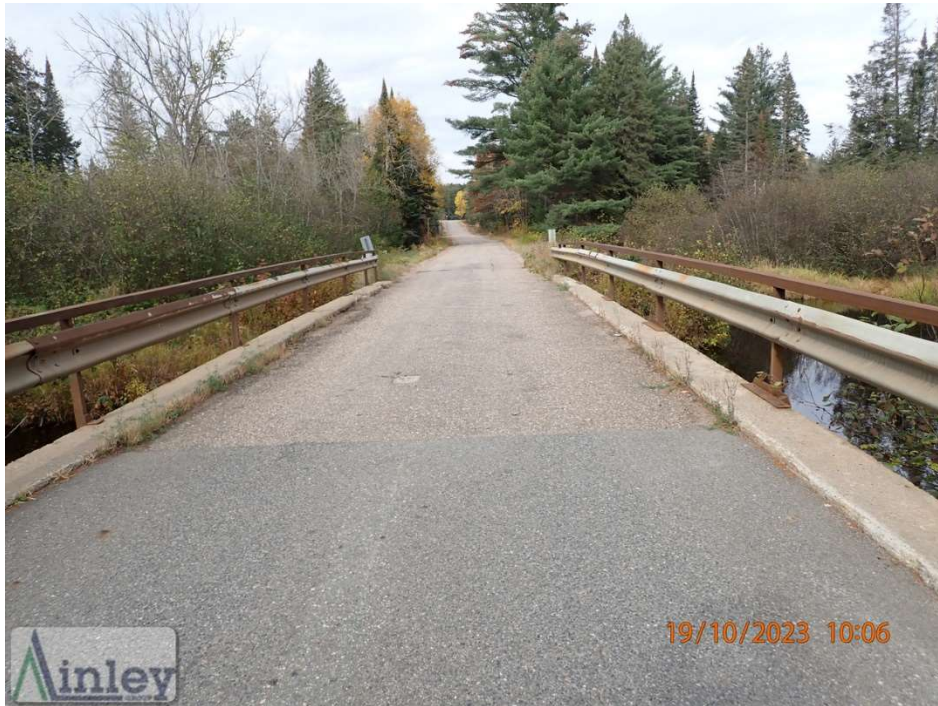
Photo 5: Deck Wearing Surface – Partially Resurfaced, Medium Ravelling and Localized Light Pothole
