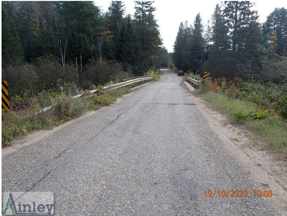
Photo 3: North Approach Looking at Structure – Medium Ravelling, Patched Potholes, Localized Severe Longitudinal and Transverse Cracks
