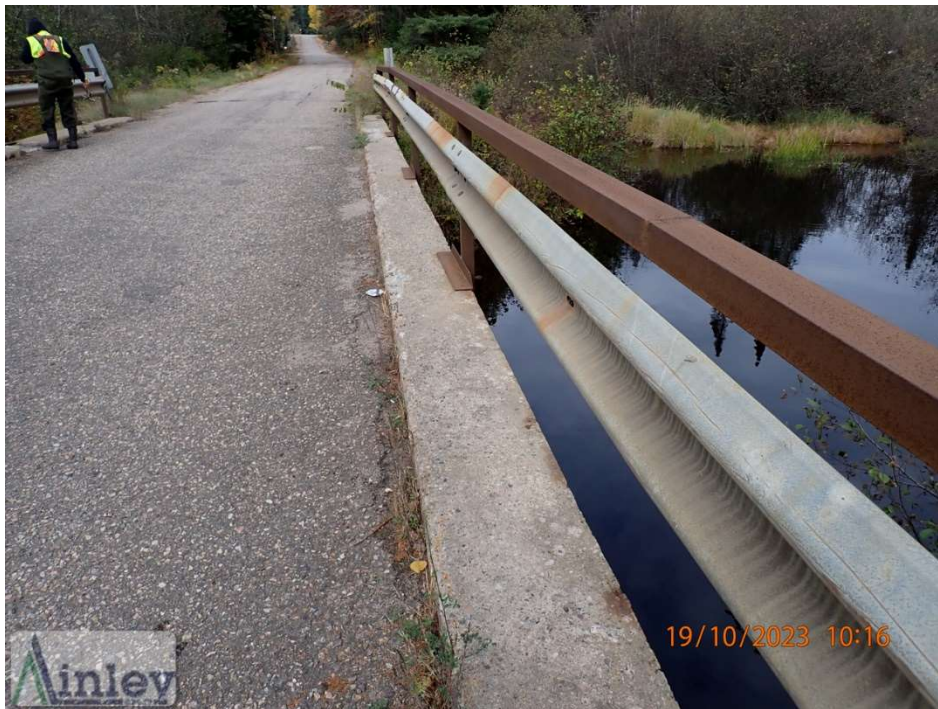
Photo 8: East Curb – Light Scaling Throughout, Localized Light Spalls and Light to Medium Cracks
