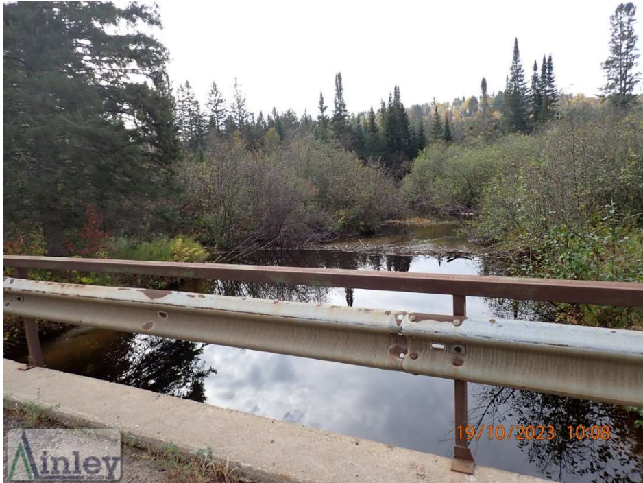
Photo 7: West Railing System – Light Corrosion Throughout Handrail and Posts, Sporadic Light Corrosion in SGBR
