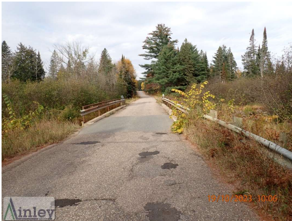
Photo 4: South Approach Looking at Structure – Medium Ravelling, Patched Potholes, Light to Medium Cracks Throughout
