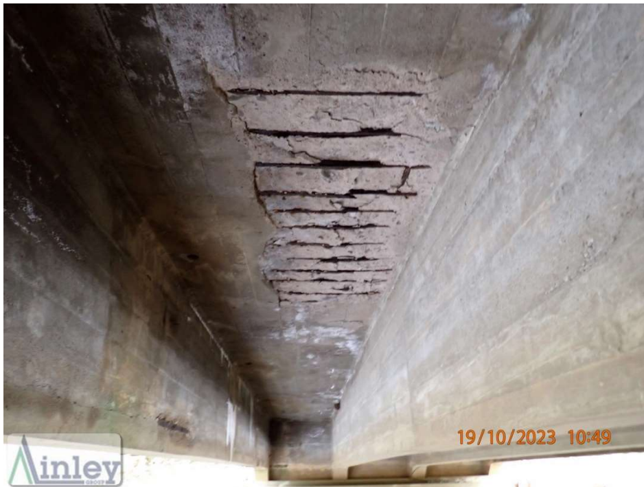
Photo 12: Deck Soffit Looking South – Delamination and Spalling with Exposed Corroded Rebar
