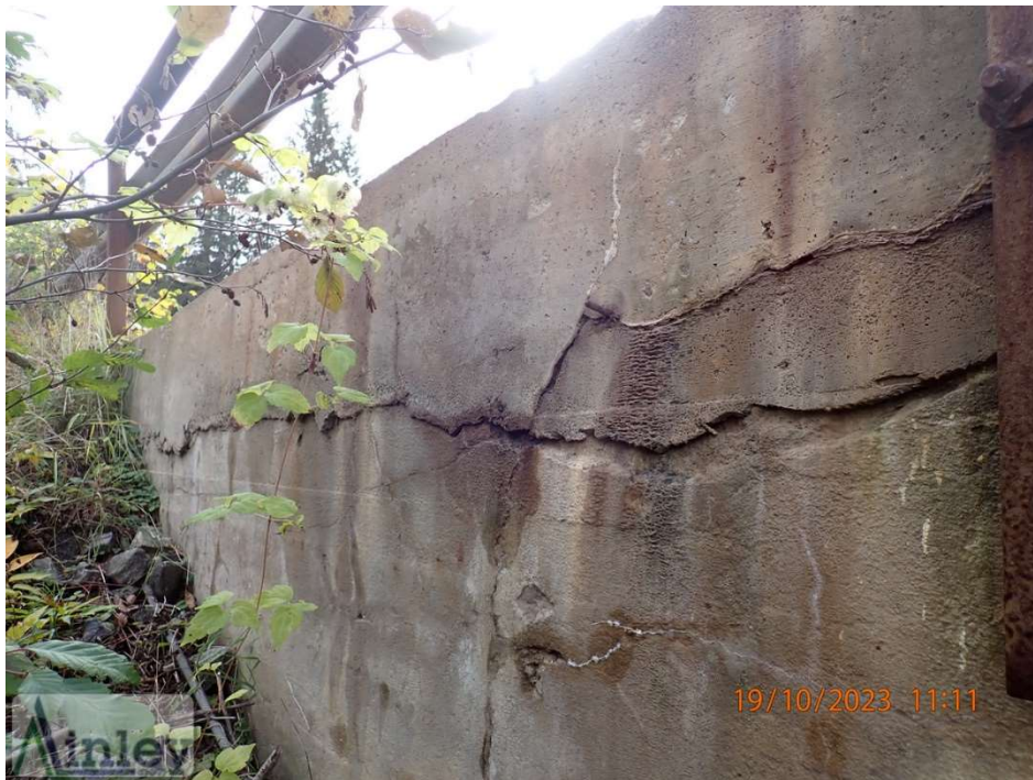
Photo 18: Southeast Wingwall – Wide Horizontal and Vertical Cracks with Moisture Staining Throughout, Cold Joint
