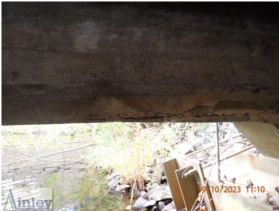
Photo 10: East Exterior Girder – Light Scaling and Wide Horizontal Crack in Interior Face of the Girder
