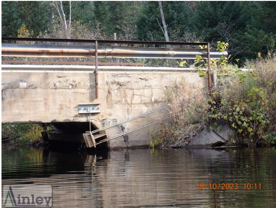
Photo 17: Southwest Wingwall – Localized Medium Spalls, Scaling and Honeycombing, Wide Horizontal and Vertical Cracks with Efflorescence and Moisture Staining Throughout
