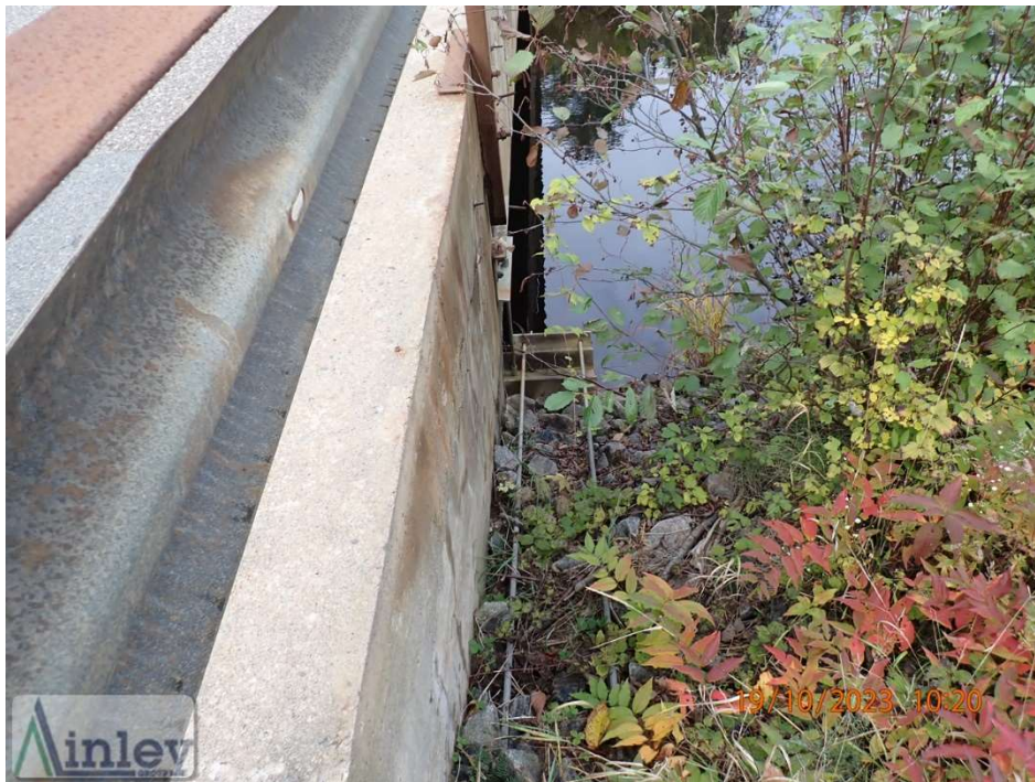
Photo 20: Southeast Embankment – Medium Erosion
