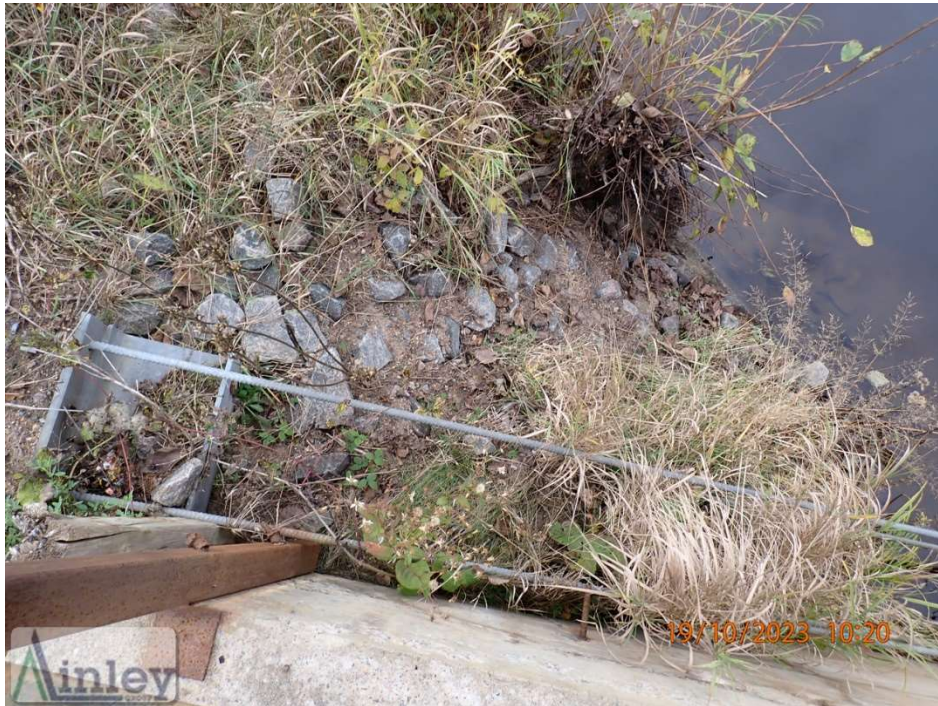
Photo 19: Southwest Embankment – Medium Erosion
