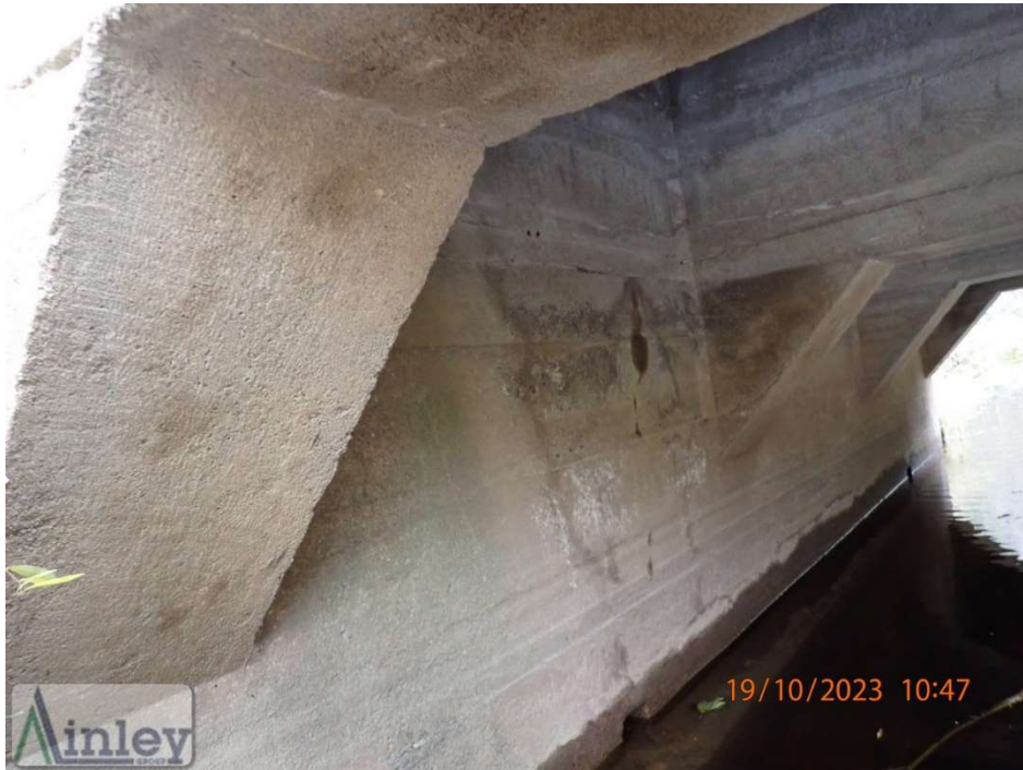
Photo 13: North Abutment Wall – Light Scaling Throughout, Localized Efflorescence and Moisture Staining
