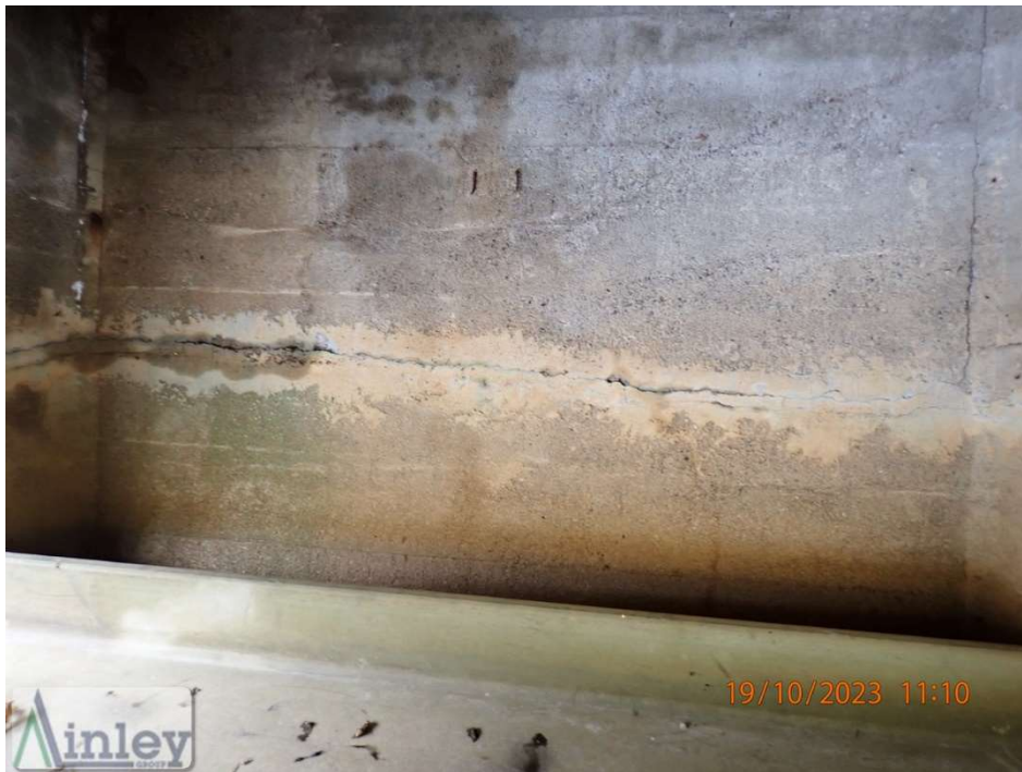
Photo 14: South Abutment Wall – Light Scaling Throughout, Moisture Staining and Localized Wide Crack Throughout the Length of the Wall
