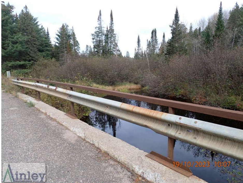
Photo 6: East Railing System – Light Corrosion Throughout Handrail and Posts, Sporadic Light Corrosion and Localized Collision Damage in SGBR
