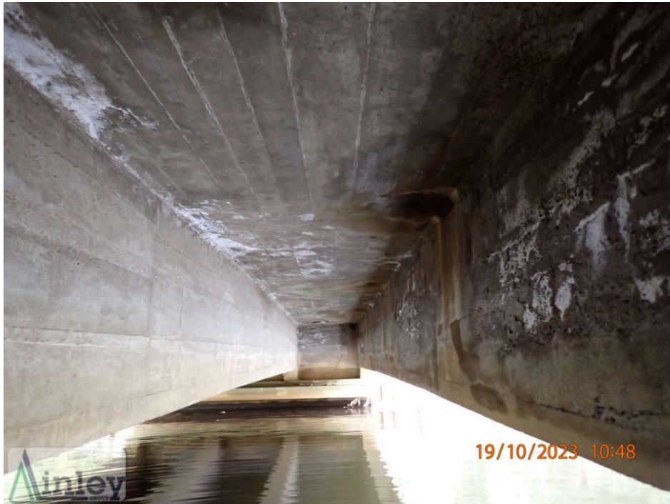
Photo 11: Deck Soffit Looking South – Efflorescence and Moisture Stains, Localized Light Scaling
