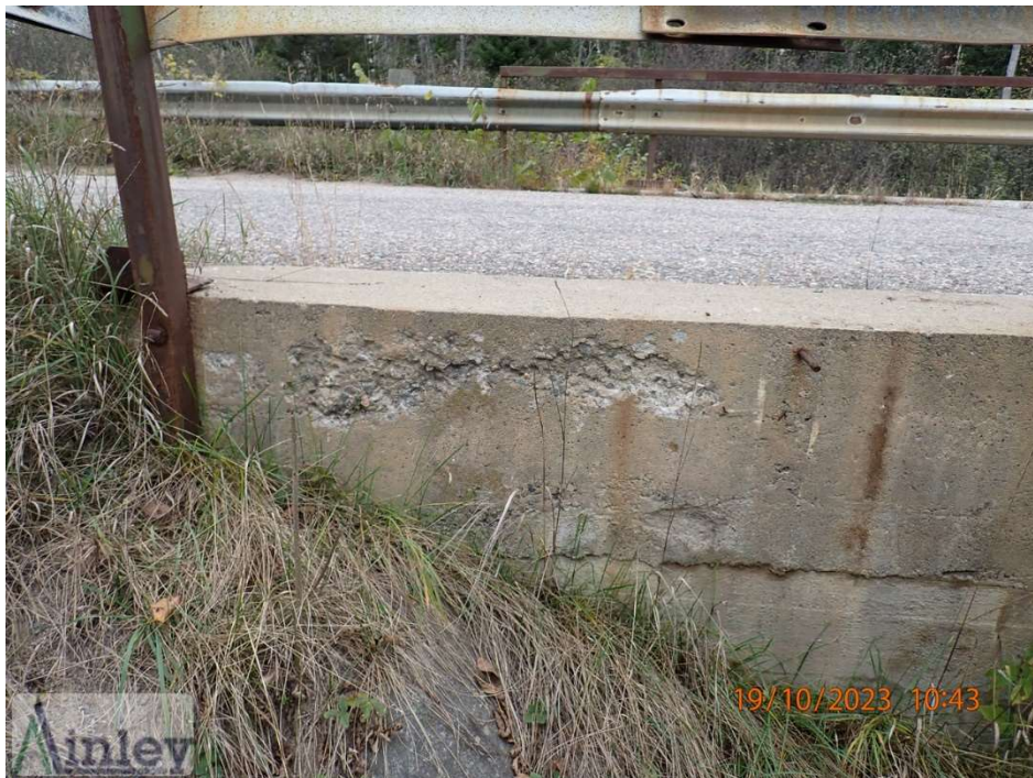
Photo 16: Northwest Wingwall – Localized Medium Spalling, Cold Joint, Moisture and Rust Staining
