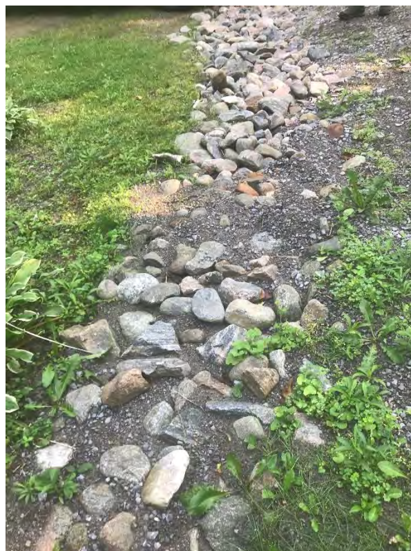
Photo 6 – Existing “French Drain” system at 3248 Papineau Lake Road (August 24, 2021).
